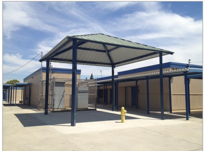
2. Installation of the new shade structure at the northwest side of the campus.-Phase Nine
