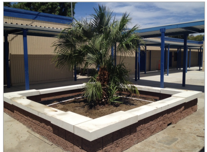
4. Completed concrete masonry unit planter and seat caps, with irrigation and landscape placement on going.-Phase Nine
